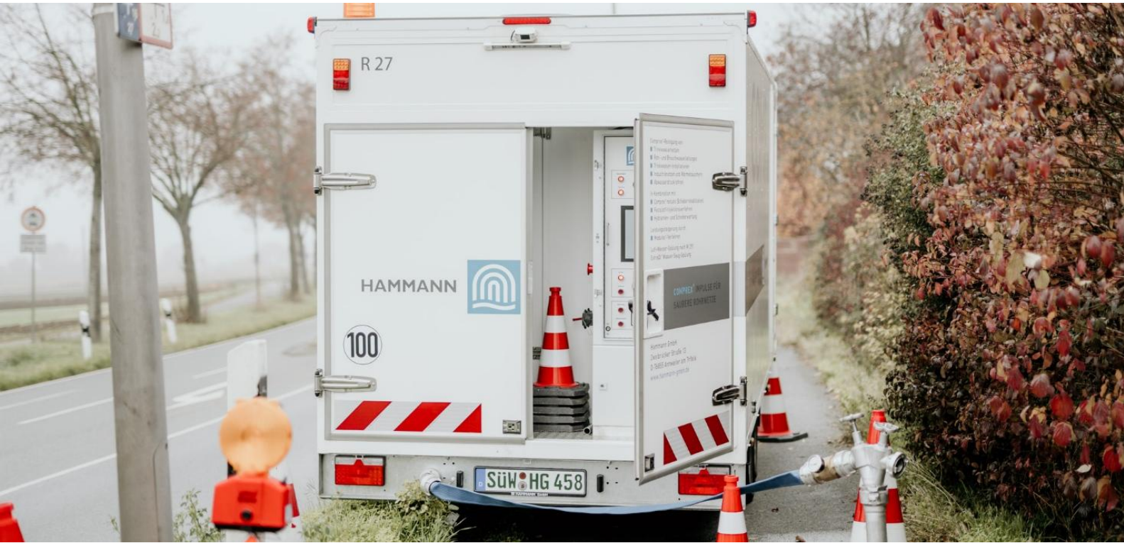
Figure 4: complex unit at the feed point
