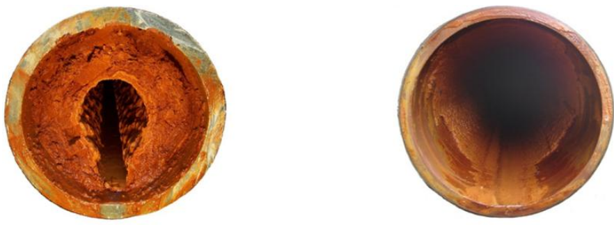
Figure 11: Raw water pipeline made of asbestos cement before and after complex impulse cleaning
