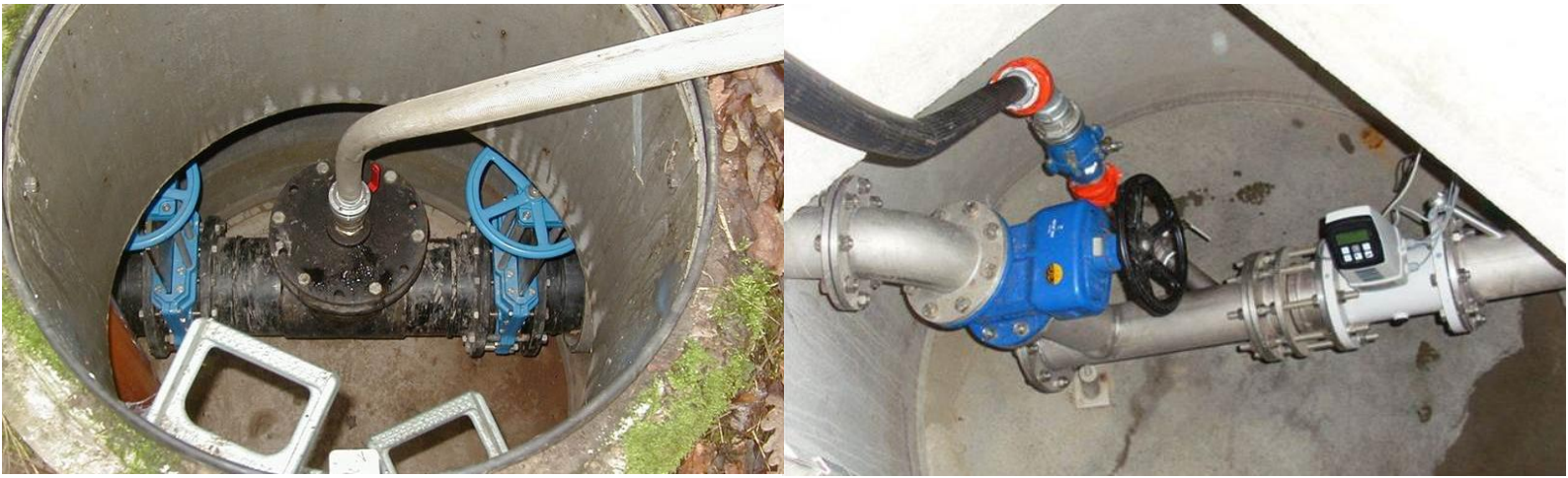
Figure 6: Inlet points for compressed air in wastewater pressure lines at air valve or drain points
